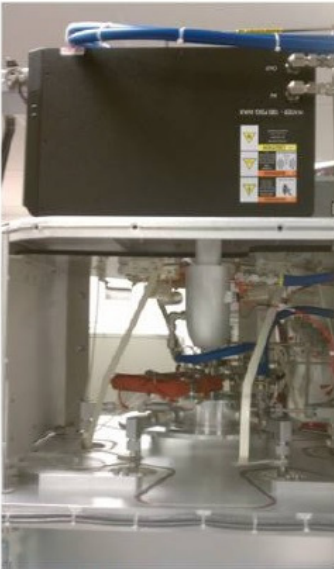
C1 RPC Generator Location
